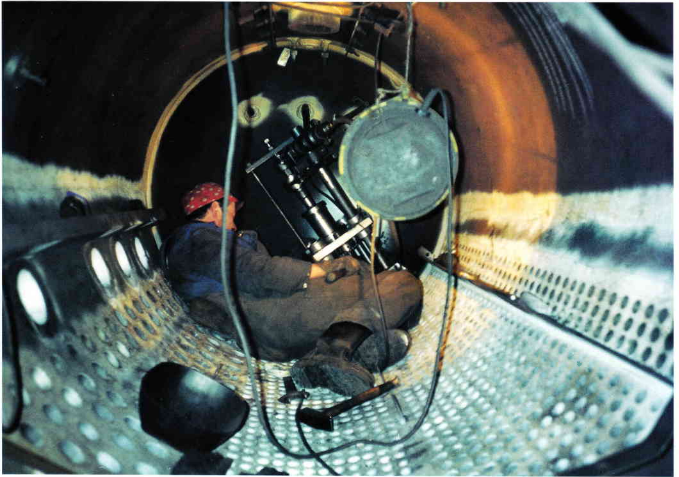
Steam drum repair: Machining tool for boring the penetration for renewal and welding of new down comer tube stubs
