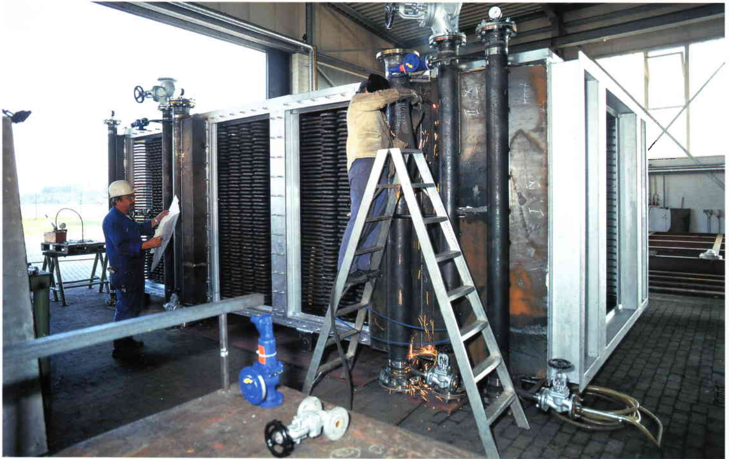
Exhaust gas boiler fabrication: Plain tube type exhaust gas boiler, weight 60 tons, during completion. The unit was designed and made to replace a totally burnt exhaust gas boiler of finned tubes on same outer dimensions and connections for a turnkey and easy refit
