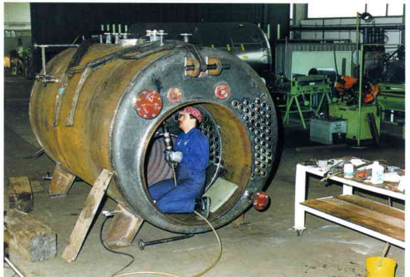
Auxiliary boiler for container ship, fabrication of entire pressure parts as per sample for replacement on board during a five days regular docking.
